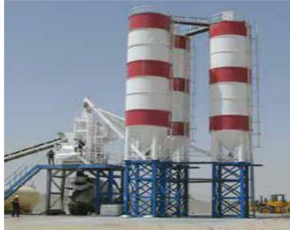
Concrete Batching Plant no.1
