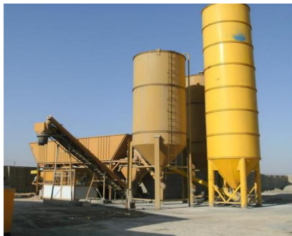
Concrete Batching Plant no.2
